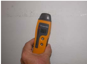
Moisture meter confirming elevated moisture in suspect material.
